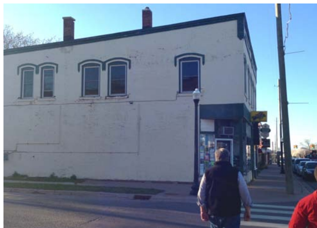
This classic building is underutilizing its side elevation. As an interim step, a mural could be painted in this area.
